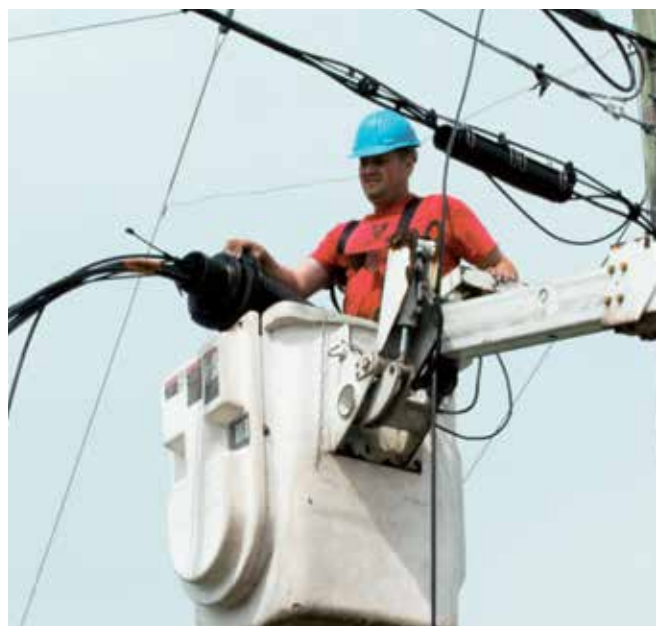
Danville, Virginia's use of its own utility poles for the nDanville network saved the city time and money.
