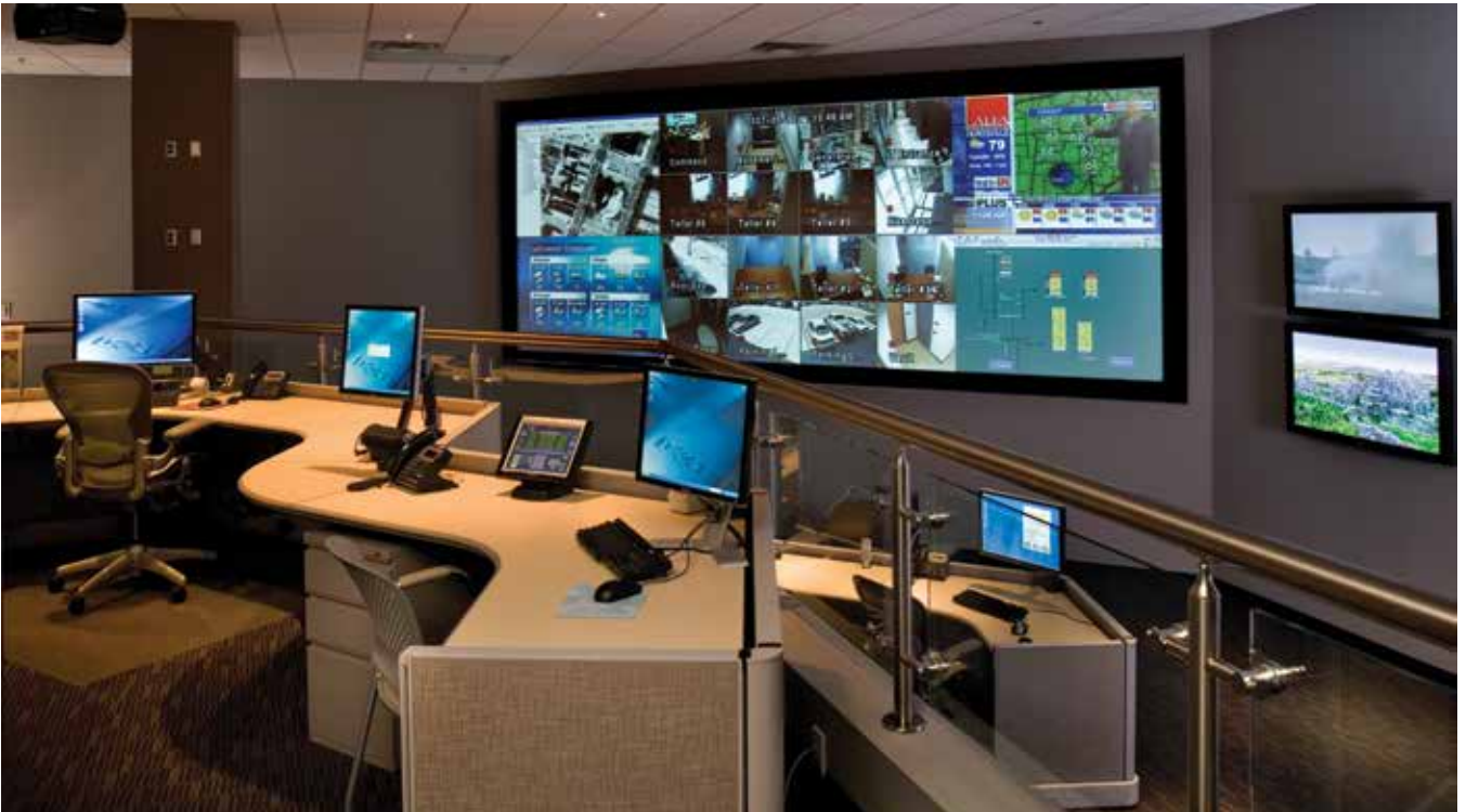
Pulaski Electric System, a municipal electric utility in Pulaski, Tenn., uses its FTTH network to operate a smart electric grid and deliver triple-play services to residents.
